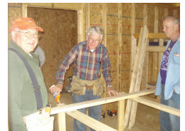
Members of State College Presby. and Derry Presby. lend a hand in construction
